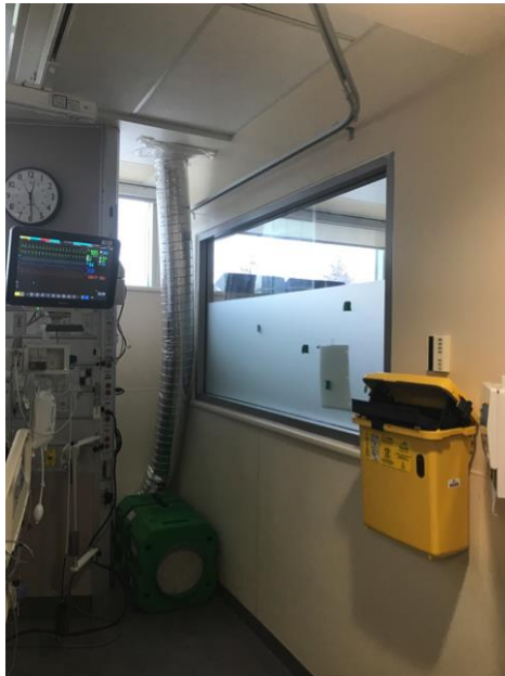
HEPA filtration with direct flow outside room
